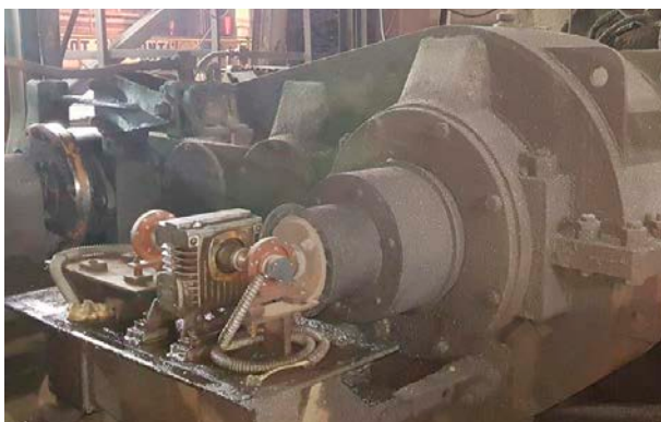
Before: Mechanical cam limit switch and absolute encoder mounted by using an additional distribution gear.
