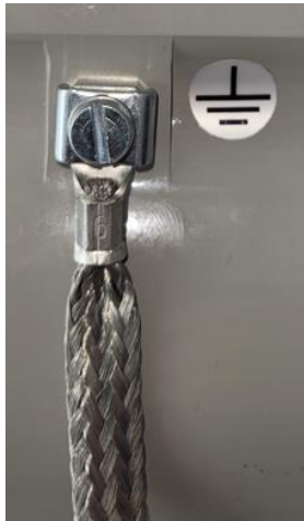
Figure 5: Permanently connected grounding strap on the USL 42 basic unit
