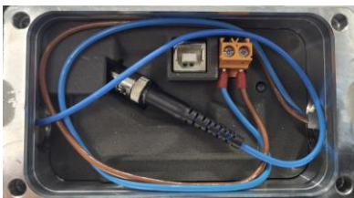
Figure 11: Fiber optic cable and supply cable in the terminal box of the USL(H) 42 basic unit
