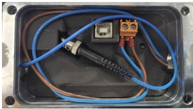
Figure: Fiber optic cable and supply cable in the terminal box of the FG 40
