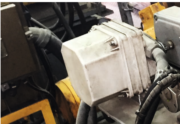
替换前: 机械凸轮限位开关. Before: Mechanical cam limit switch.
