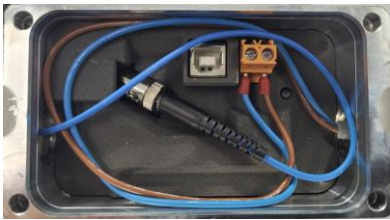
Figure 11: Fiber optic cable and supply cable in the terminal box of the USL(H) 42 basic unit
