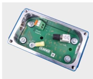
端子箱内 FOC 接头 FOC connector in a terminal box
